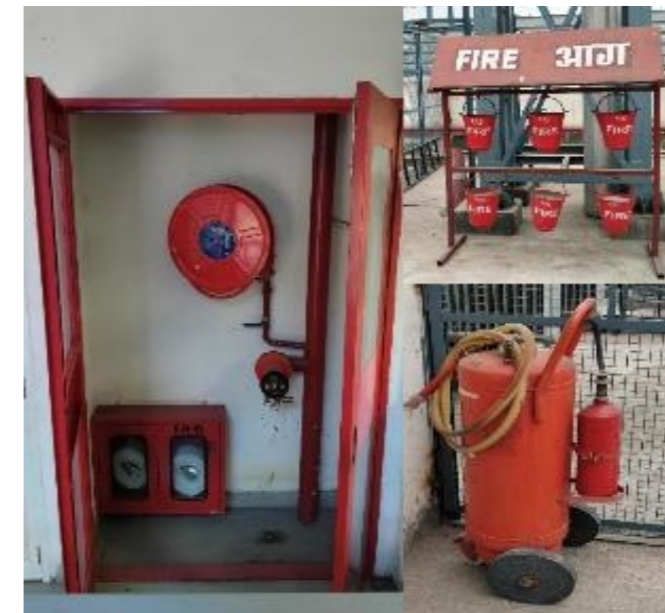
Fire Safety equipment
